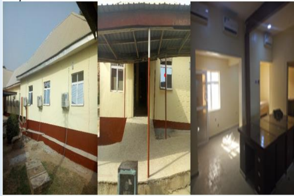
Refurbished/upgraded PCR Lab
